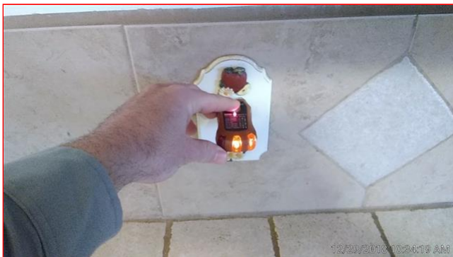
9.9 Not GFCI Protected
