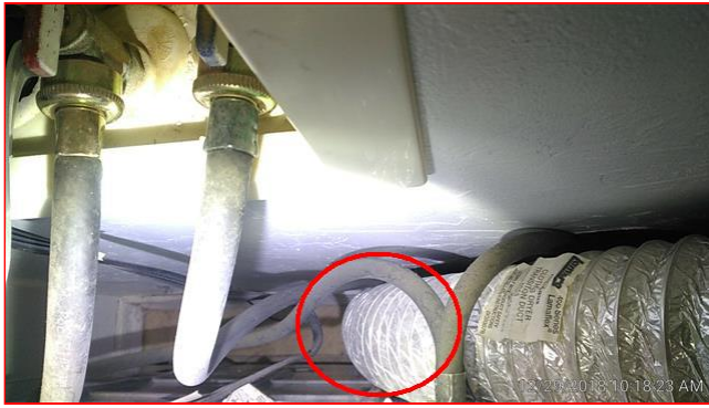
10.4 Dryer Vent Separated
